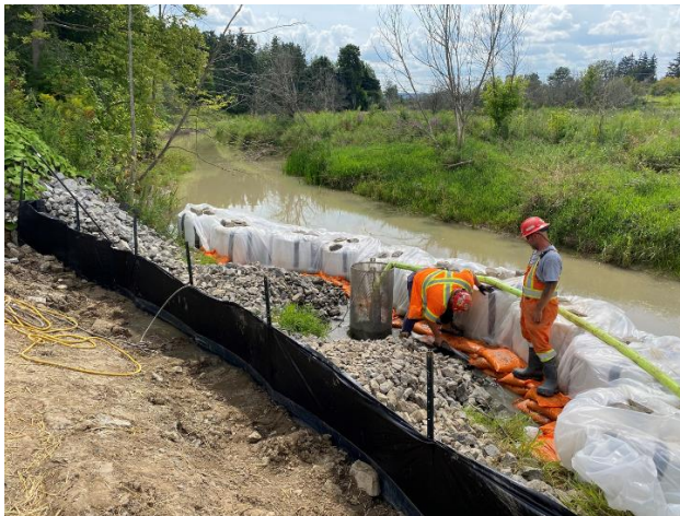
Image 1: Cofferd Dam installation and fish rescue at outlet of spillway within the Indian Creek backwater channel
