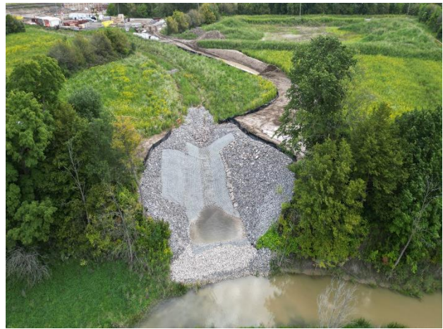
Image 4: Completed remedial work to the spillway prior to temporary access road being decommissioned and restored
