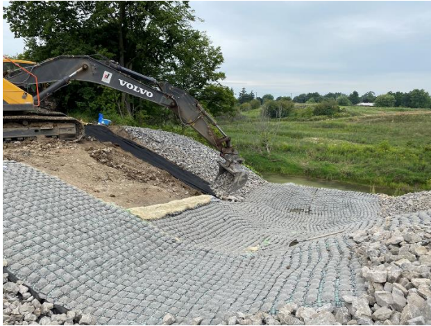
Image 3: Installation of filter cloth and rip-rap material along the banks of the spillway
