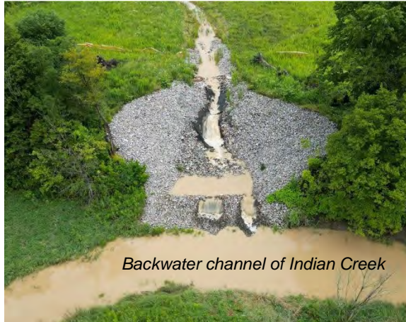
Photo 1: Spillway slope failure
