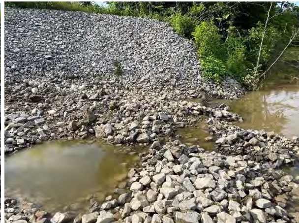
Photo 4: Displaced rip-rap deposited in plunge pool
