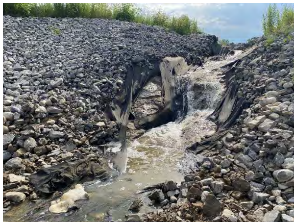
Photo 3: Exposed and torn geotextile fabric
