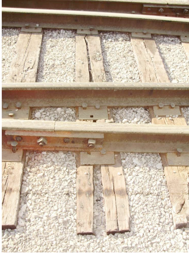
(Figure 16: Picture of split tie)
