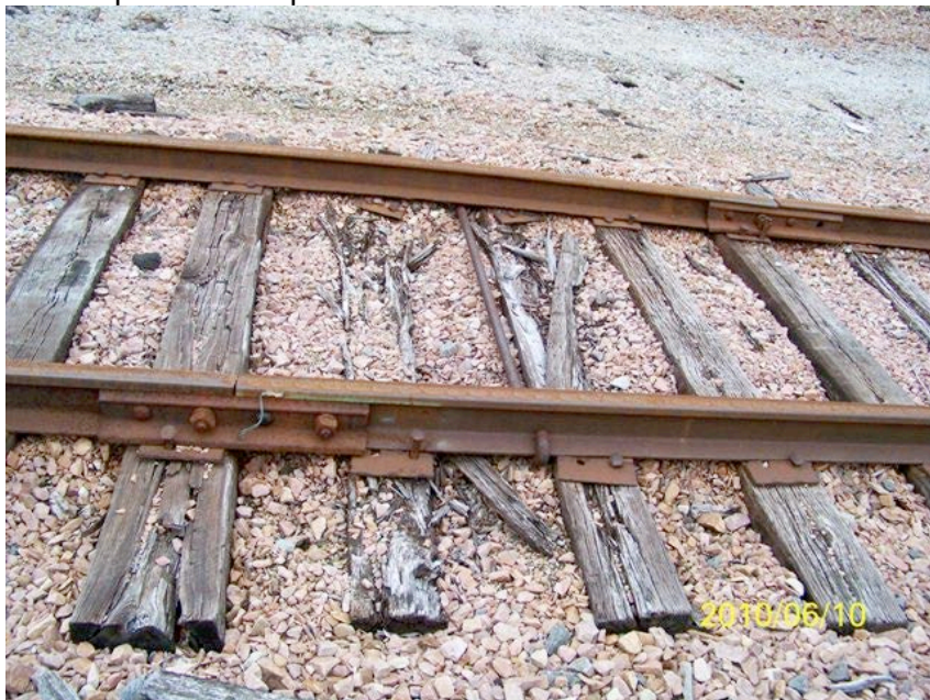
(Figure 17: Deteriorated tie)
