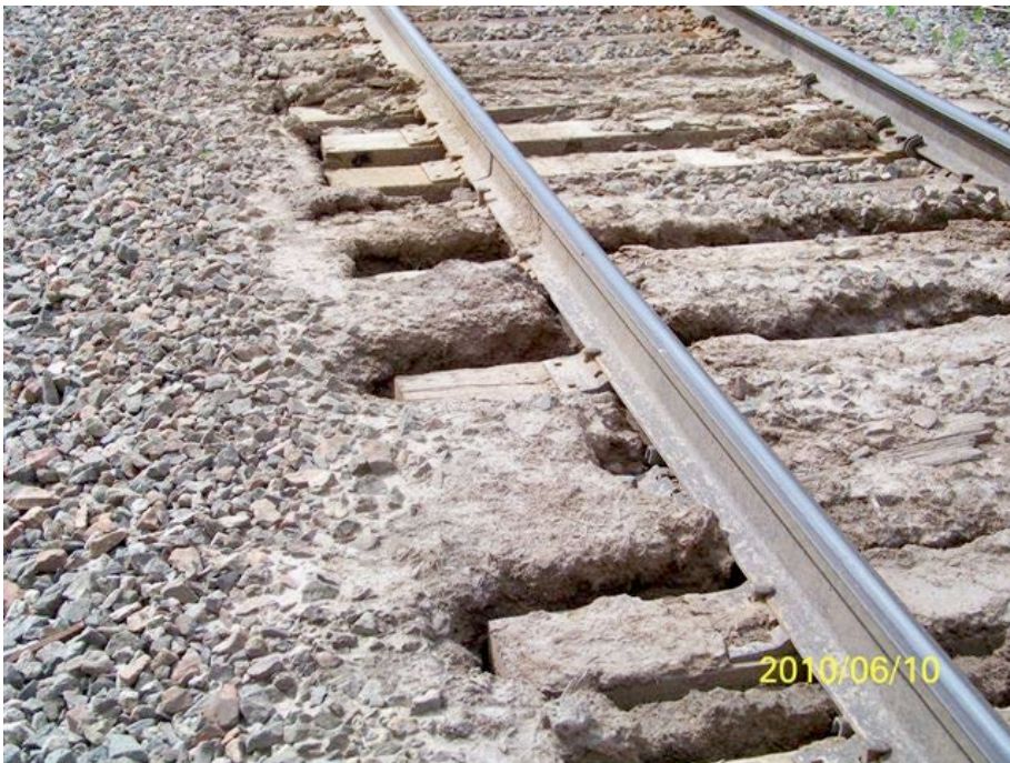
(Figure 13: Fouled and muddy ballast)
