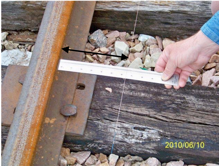
(Figure 7: More than 5 inches of movement)
