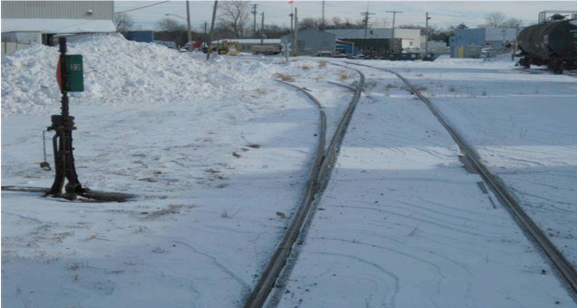
(Figure 23: Snow Packed Switch)
