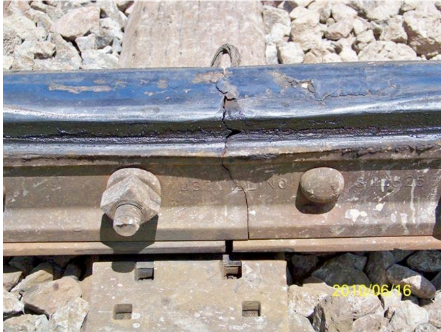
(Figure 20: Cracked joint bar)
