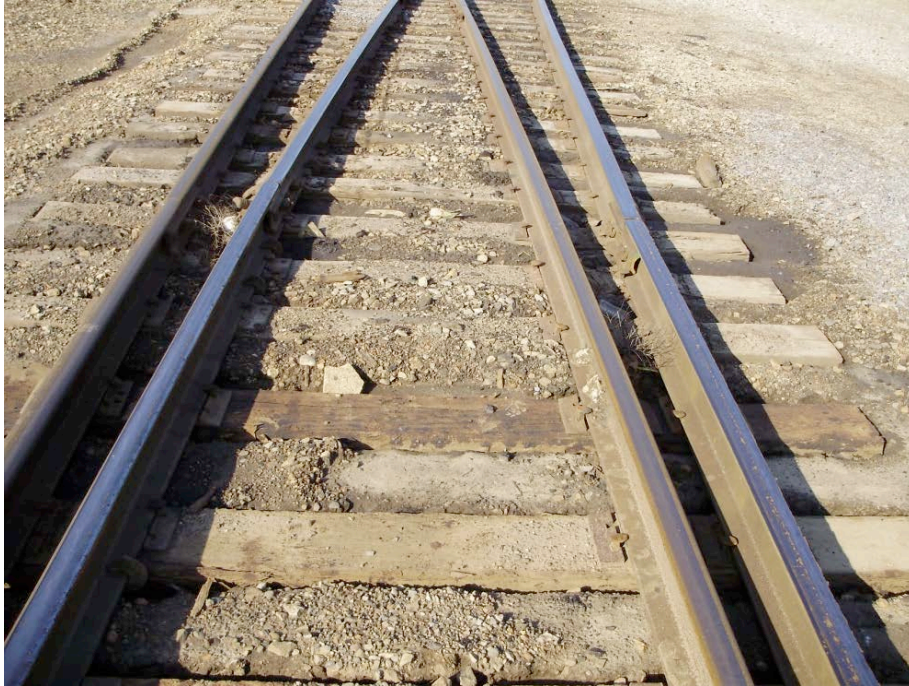
(Figure 12: Fouled and muddy ballast)
